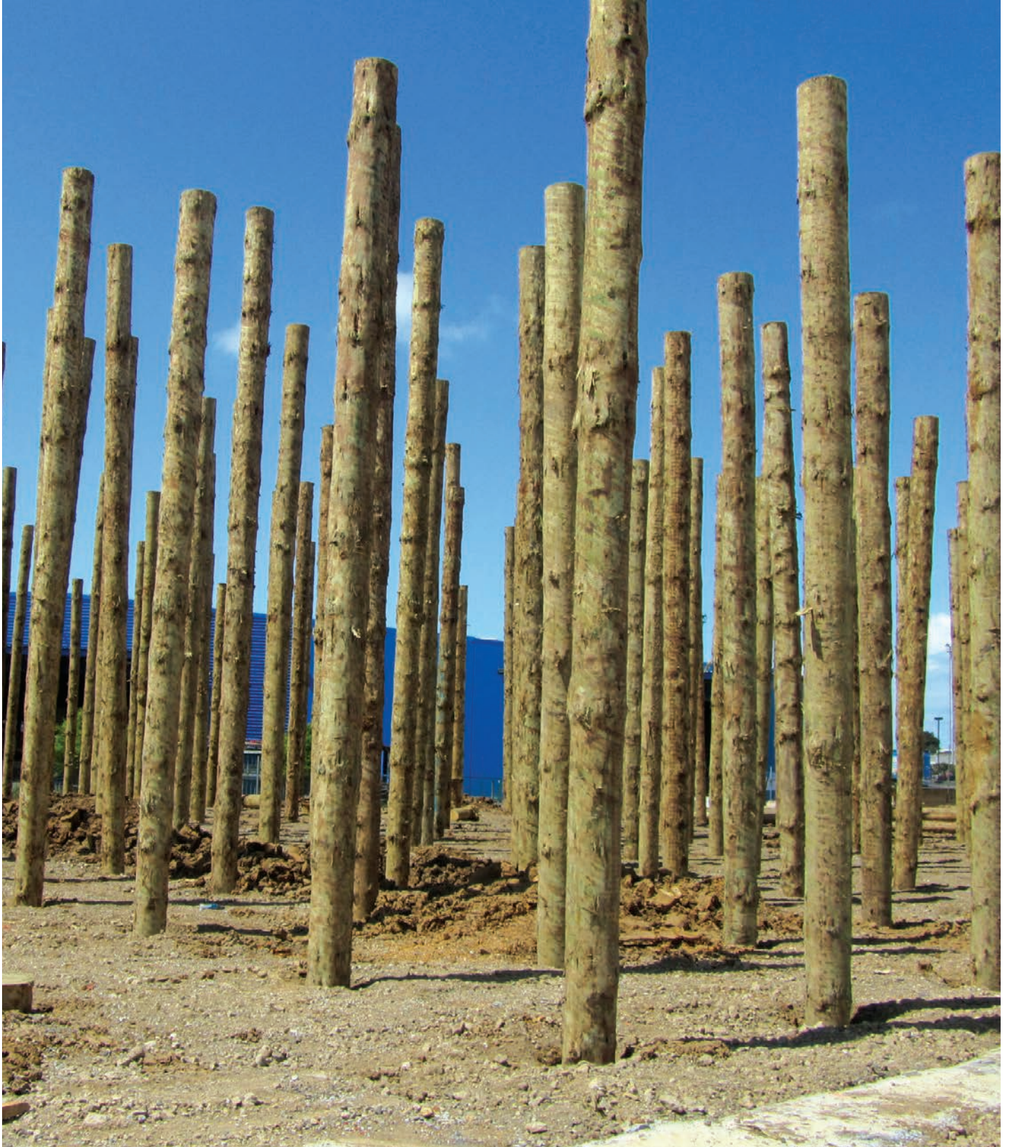
Ground improvement can be achieved by installing driven or vibrated, treated Radiata Pine poles at close centres. The above TTT H5 SED Ø300 x 9.0m Uglies were installed by pre-drilling 2.0m deep holes in both clay and silt, then standing the poles vertical and simply driving to ground level.
